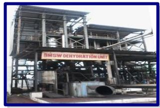
BMSW EVAPORATOR-II & ATFD
