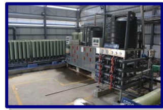
BMSW RO PLANT
